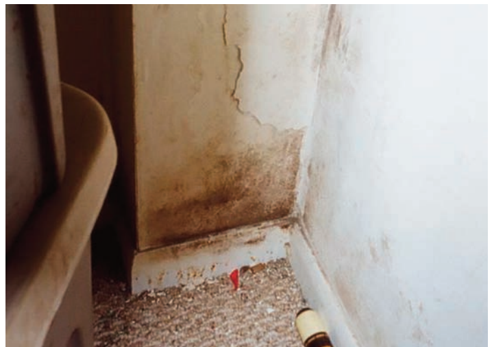
Rockwell Gardens Construction Quality Issue: Mold in Unit Interior
